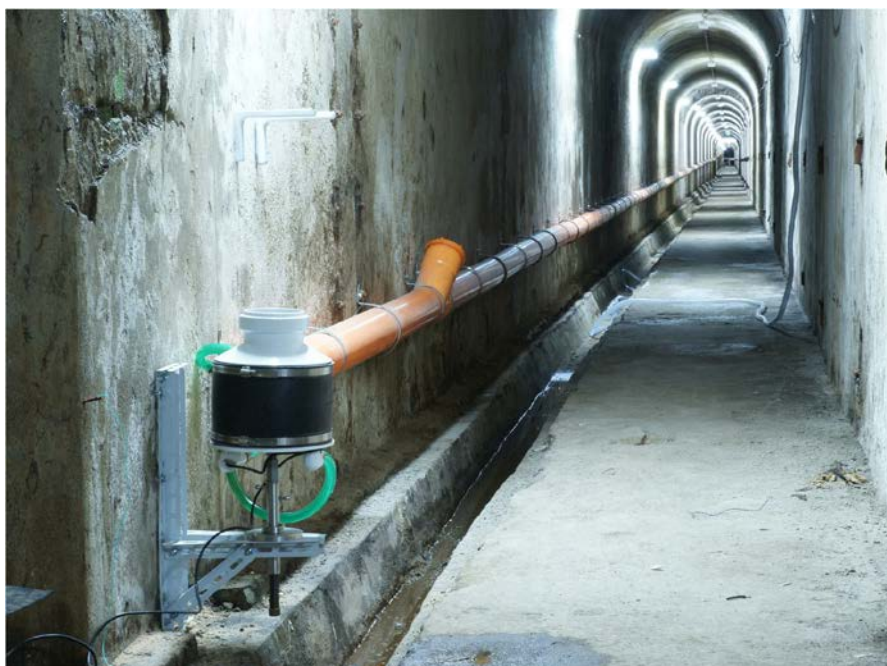
Figure 3.16 – In this picture it is shown the North tiltmeter installed near Pozzuoli: on the wall it is visible the pot where the NN sensor is installed. Picture points southward.
