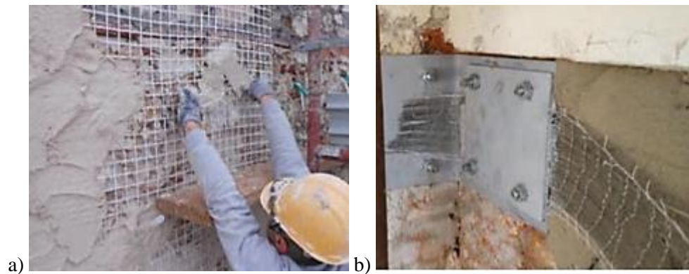
Figure 2.2: a) Reinforcement of a masonry wall by means of TRMs; b) TRM-steel mixed intervention to upgrade a masonry element capacity [10].
