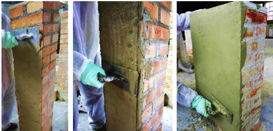
Figure 2.23: Application of the Flax-TRM system on masonry structural elements: a) application of the first layer of mortar; b) embedding of the fabric into the matrix; c) smoothing of the outer layer of mortar [86].
