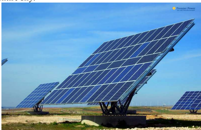
Figure 21 – Tracking array system.
