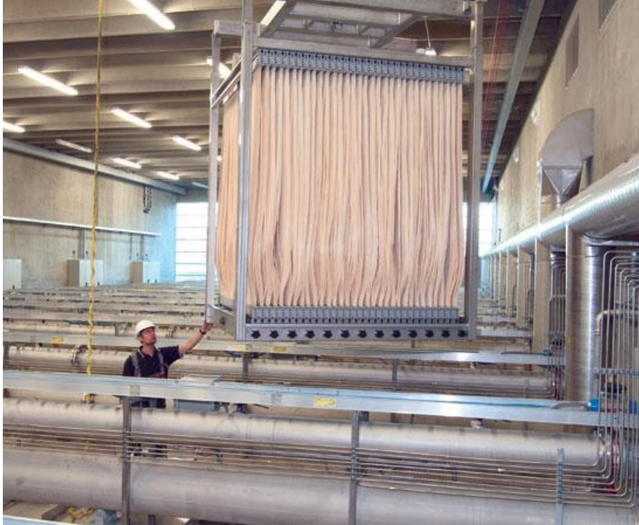
Figure 1-3 - Membrane BioReactor installation (courtesy of GE Water, US)
