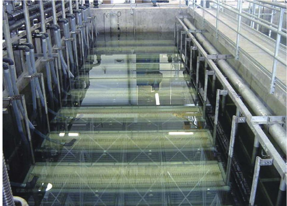
Figure 2-2 - MBR chemical cleaning, in which the modules are soaked into a sodium hypochlorite solution (courtesy of Ovivo, Australia)
