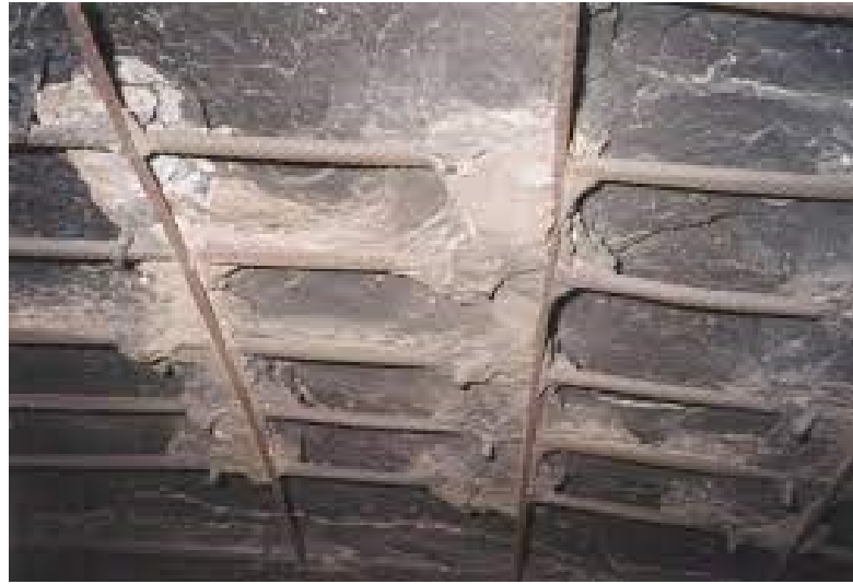
Fig. 1.4. Concrete element affected by spalling ( Mastronardi, 2013 ).
