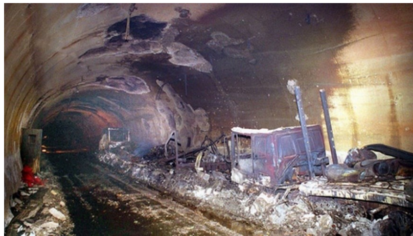
Fig. 1.1. Mont Blanc tunnel fire in 1999 with 39 depths.
