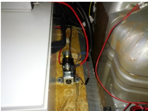
Figure 3.6 - Installed battery pack contactor
