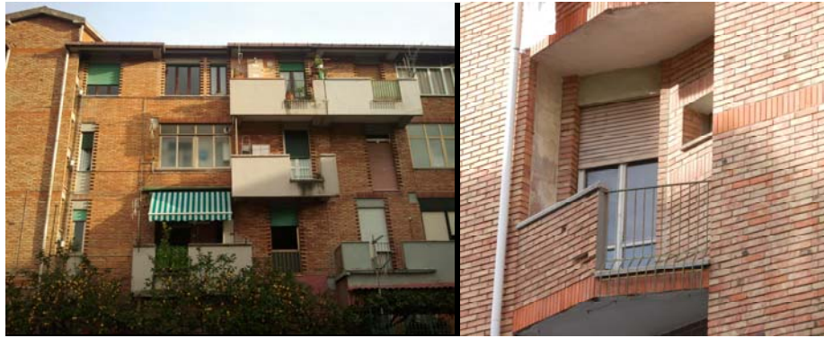
Fig.4. 20: As can be seen from the picture, each owner did autonomous maintenance interventions, there is no homogeneity. Quartiere Pastena , Bruno Zevi Salerno.
