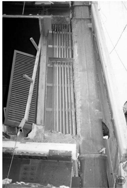
Fig. 2.13 – Failure of beam-to-column fillet welded connection (Kobe Earthquake)
