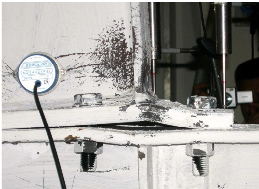
Fig. 3.36 – Formation of the crack in the end-plate
