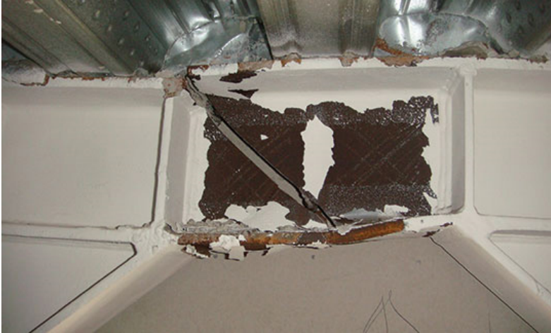
Figure 1.4 – EBFs with K-scheme damaged during Christchurch Earthquake (2011)
