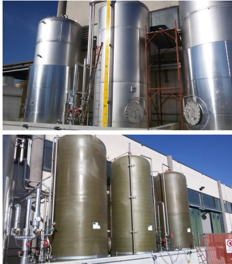
Figure 81. Storage tanks area
