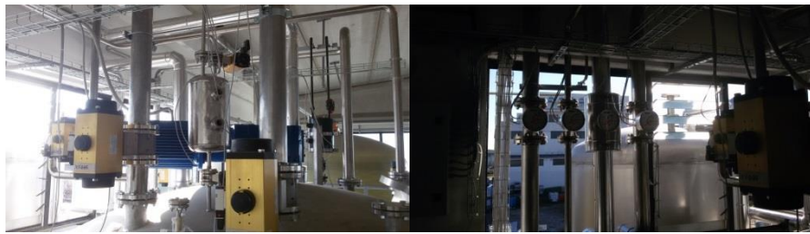
Figure 85. Detail of the top of reactor (on the left) and flow meters (on the right)
