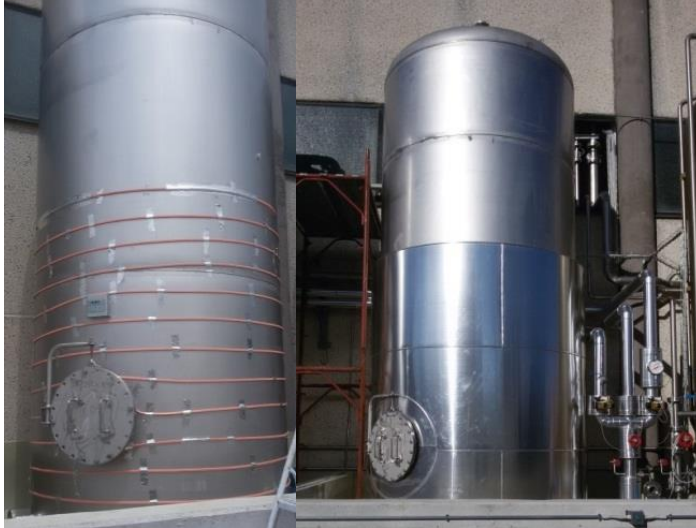
Figure 82. Phenol storage tank before (on the left) and after (on the right) insulation
