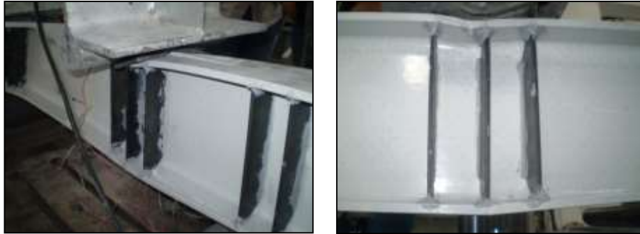
Figure 4.9. Local cracks in T1_1.
