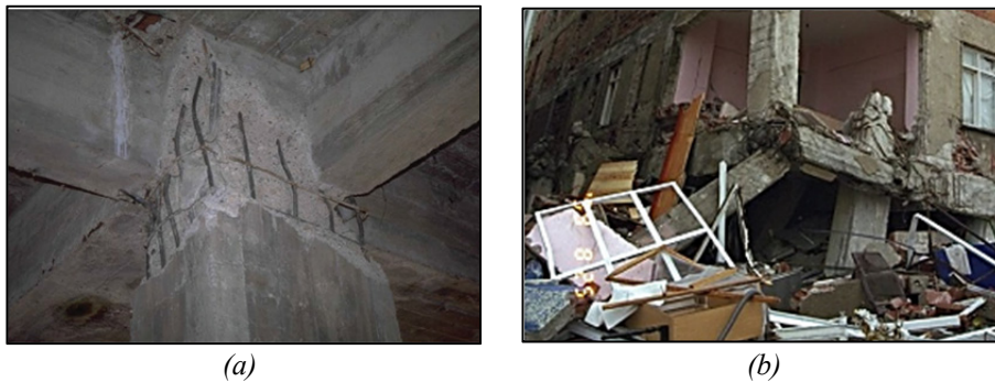
Figure 1.5: a) Poor beam-column connection; b) failure of a corner joint
