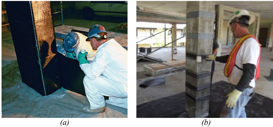
Figure 3.16: Example of complete (a) and partial (b) FRP wrapping of a column
