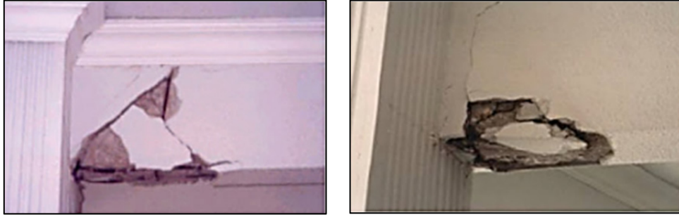
Figure 1.4: Example of shear failure in the beam [35]
