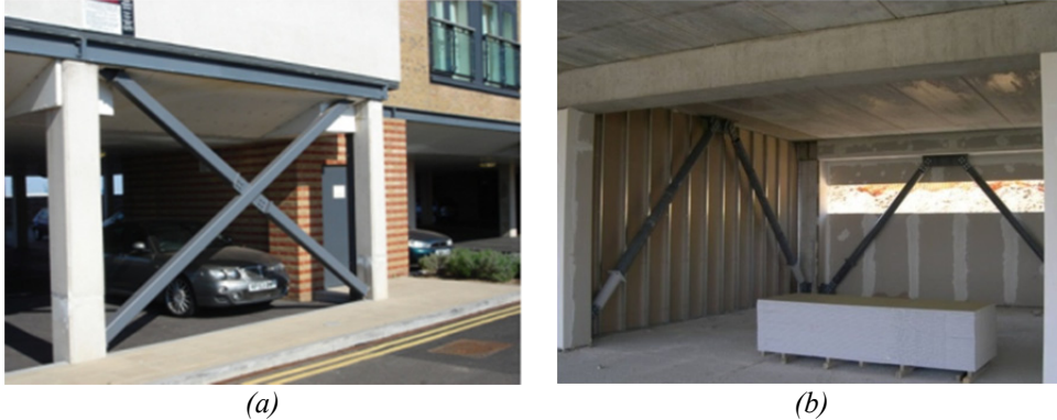
Figure 3.13: Example of steel braces installed on the ground floor (a); with dampers (b)
