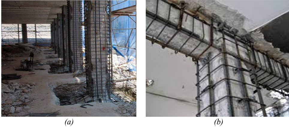
Figure 3.14: Example of concrete jacketing of columns (a); of a beam-column joint (b)
