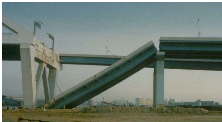
Figure 2.9: Nishinomiya-ko Bridge approach span collapse (Kobe Collection, EERC Library, University of California, Berkeley).
