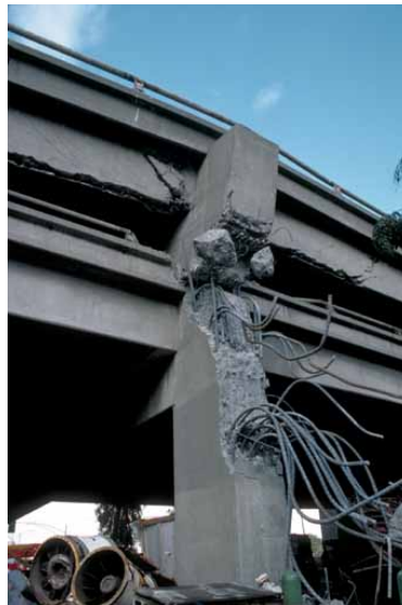
Figure 2.2: Cypress viaduct: lack of proper reinforcement in pier-deck connections. (Nakata et al. 1999)
