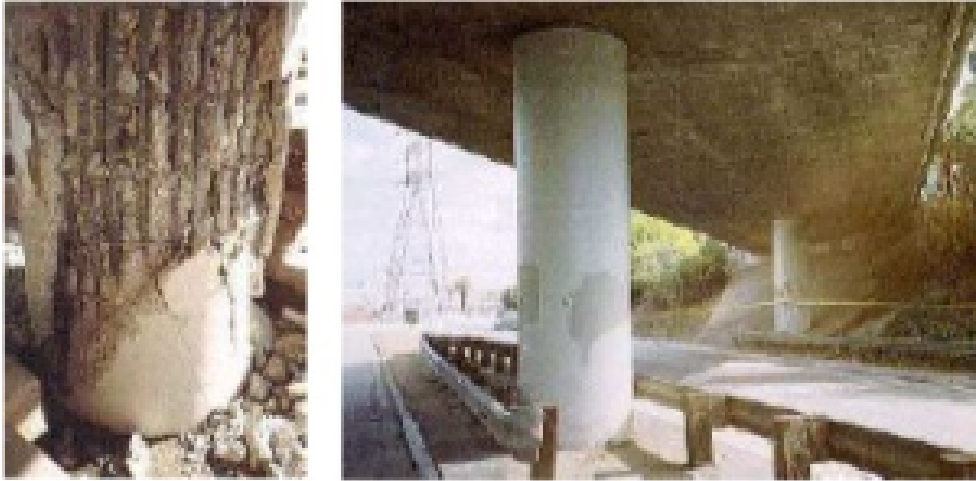
Figure 2.6: Failure of the column due to the failure of circular confinement steel (left); good behaviour of column retrofitted (right). (Todd et al. 1994)
