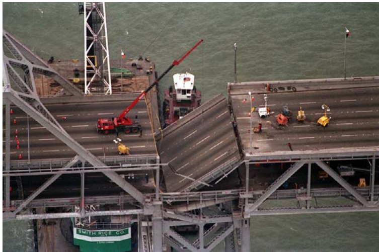
Figure 2.3: Oakland Bay Bridge: a collapsed portion of the upper deck. (Nakata et al. 1999).
