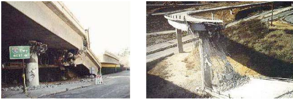
Figure 2.4: Collapsed section in Santa Monica (left) and Antelope Valley Freeway (right). (Todd et al. 1994)
