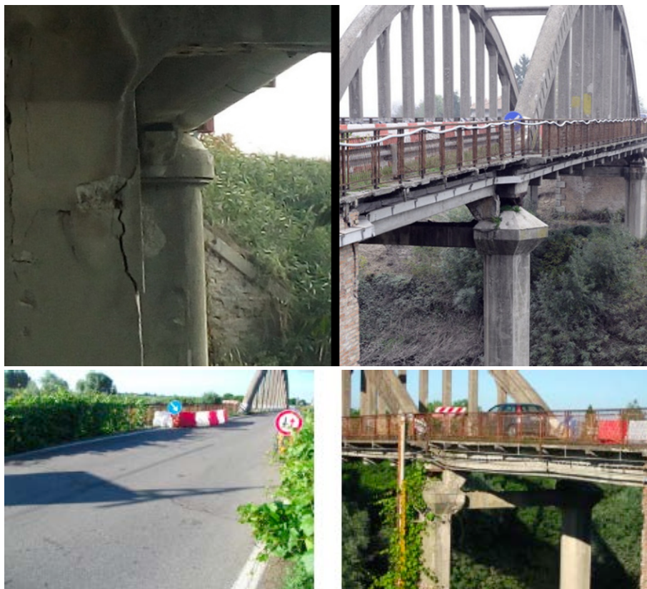
Figure 2.15: Bompoto Bridge, damage report (EPICentre Report No. EPI-FO-290512).
