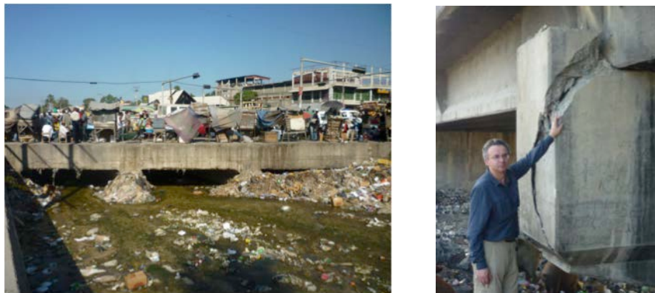
Figure 2.11: Box culvert in Port-au-Prince (left); damage to the shear key at intermediate support of bridge (right) (Eberhard et al., 2010).
