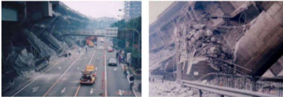
Figure 2.7: Collapsed Fukae Viaduct (left) and Premature Shear Failure of Reinforced Concrete Column, Fukae Viaduct (right) (Kawashima, 2007).
