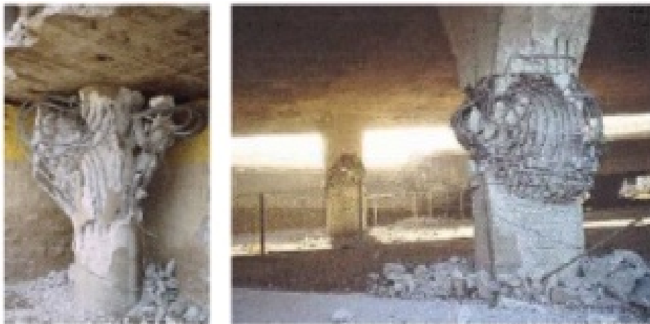
Figure 2.5: Failure of columns: insufficient confinement (left); shear failure (right). (Todd et al. 1994)
