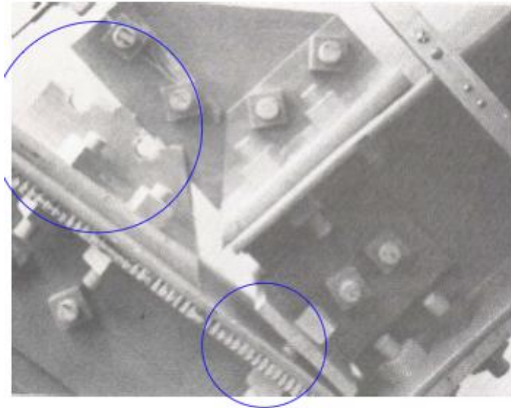
Figure 1.17. Ultimate Failure Mode of Connection Details Type iii .
