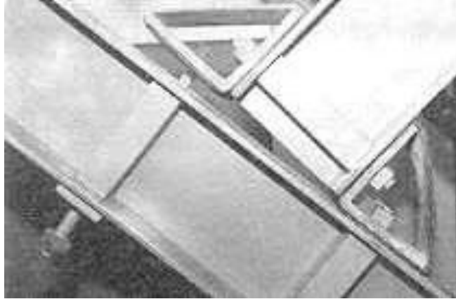
Figure 1.53. Local failure of 6" x ½" wrapped angle connection detail.
