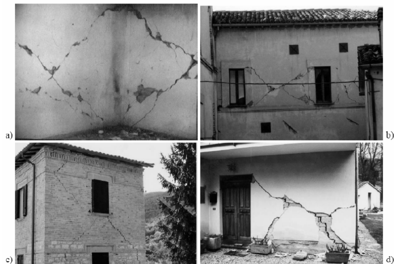
Fig. 1.14: In-plane damages of unreinforced masonry walls: a) Irpinia 1980, A.Giuffrè; b) - d) Umbria-Marche 1997 L.D. Decanini (Decanini, 2009c).
