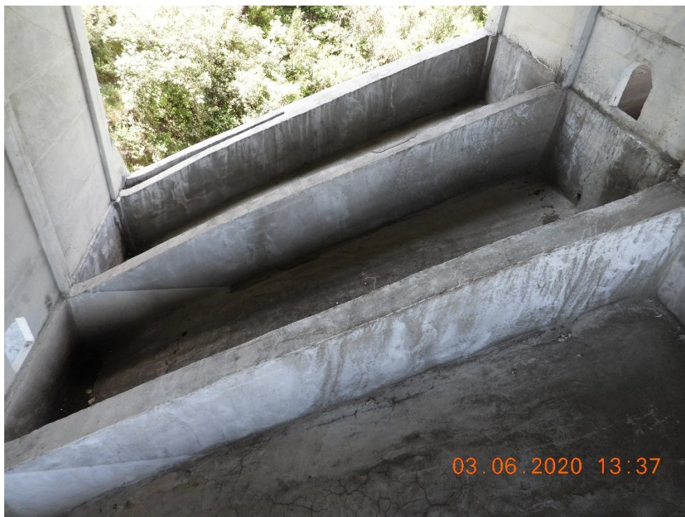
Figure 7.30 – Defects affecting the arch slab and joists of the Olivieri Viaduct [96]
