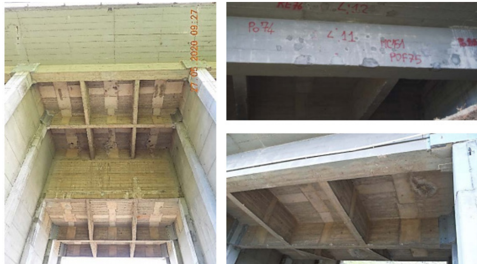
Figure 4.11 – The Olivieri viaduct registered defects affecting girders and beams [96]
