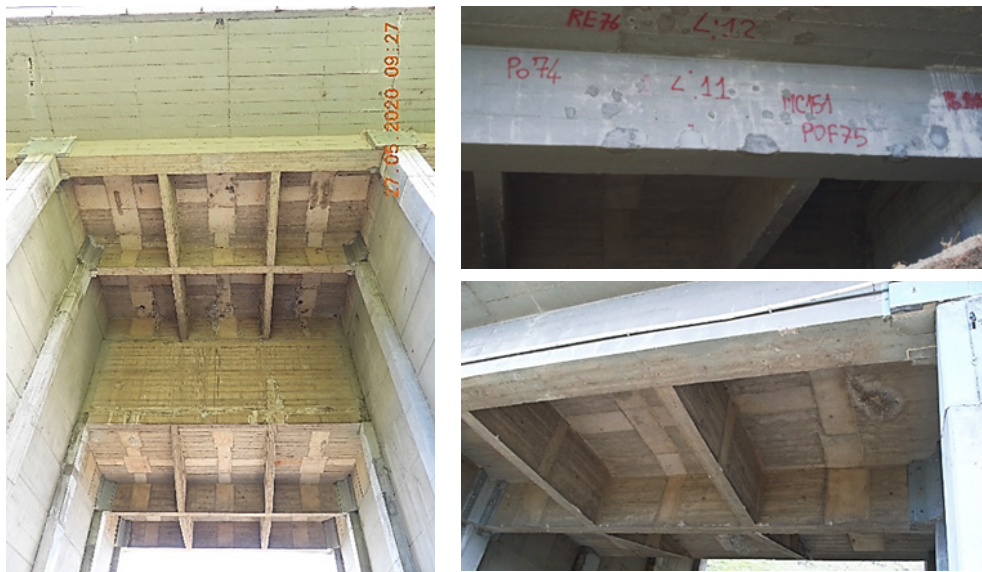
Figure 7.29 – Defects affecting the beams and joists of the Olivieri Viaduct [96]
