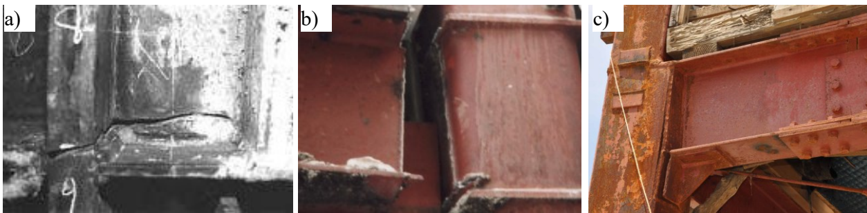
Figure 2.11. Damaged welded connections after the seismic event of a) Northridge 1994 [14-15]; b) Kobe 1995 [16]; c) Tohoku 2011 [17].
