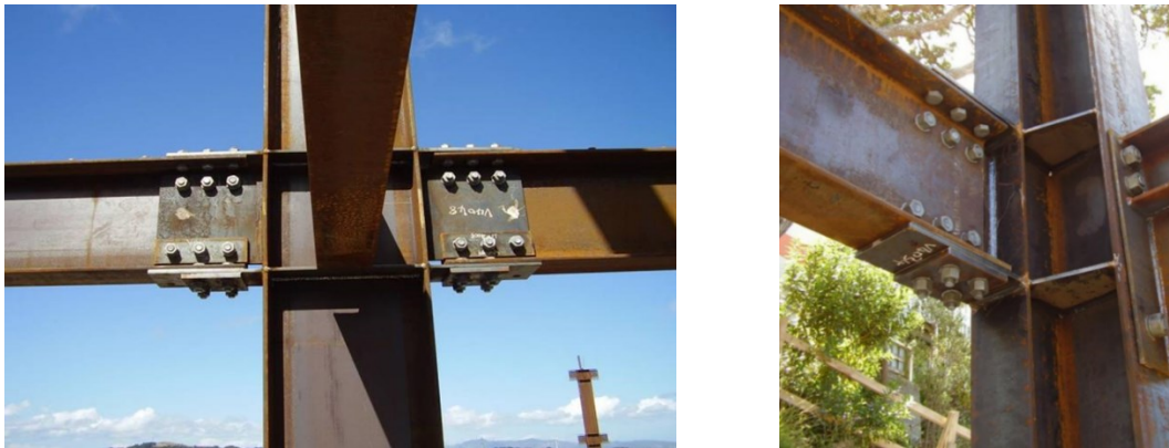
Figure 2.26. SHJ adopted in new buildings in New Zealand ( Te Puni Village Buildings ) [72-75]
