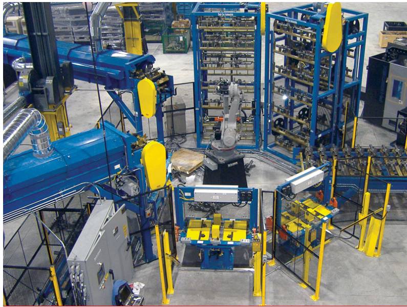
Figure 1.2 Automated Material Handling System.
