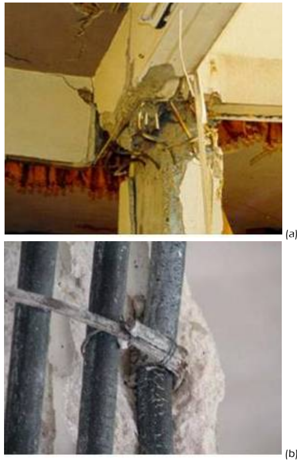
Fig. 1.1: Joint failure and wrong detail of stirrup (Bursi et al., 2009).
