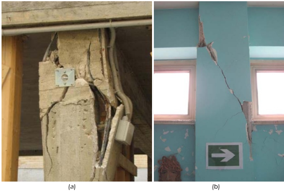
Fig. 1.4: Shear failure of squat column due to seismic events (Cimellaro, 2009).
