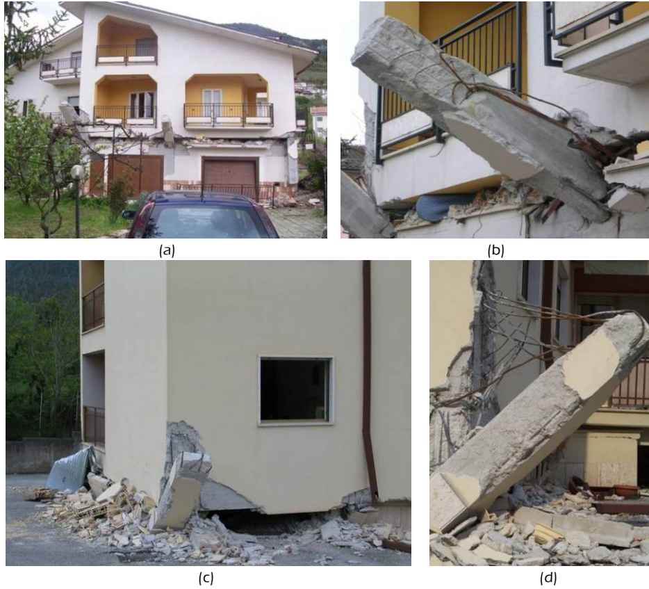
Fig. 1.2: Soft story mechanisms due to the earthquake of L'Aquila (Bursi et al., 2009).
