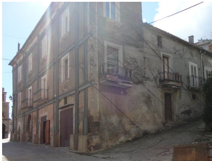
Figure 7.39: Structural interventions on building number 4 of section L-L' with damage level D5 (Peduto et al.,2017)
