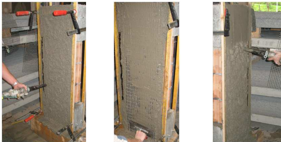
(a) Application of a layer of spray mortar (b) Embedding the carbon mesh (c) Application of another layer of spray mortar.
