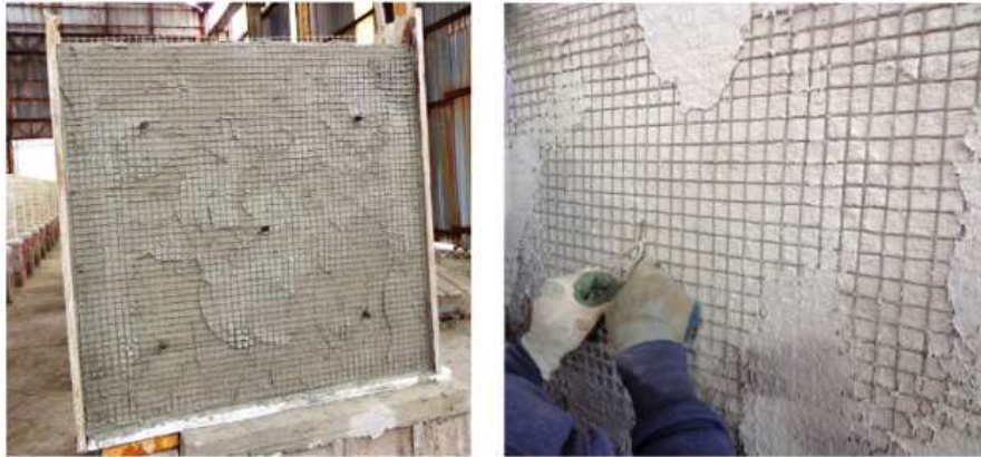
(a): Placement of one ply of HFC grid on each side of the panel (b): Installation of the anchor system on each panel side.
