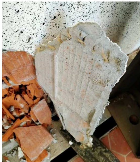
Fig. 7-45. Local collapse of a masonry structure (HBW3)
