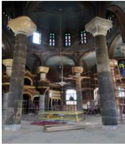
Fig. 2-55. The eight stone columns after installation of the CFRP wrapping through the columns (Hemeda 2018).
