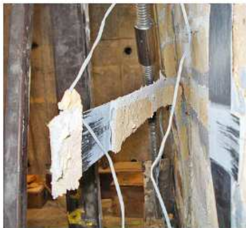
Fig. 2-56. Debonding of CFRP plate (Mahmood and Ingham 2011).
