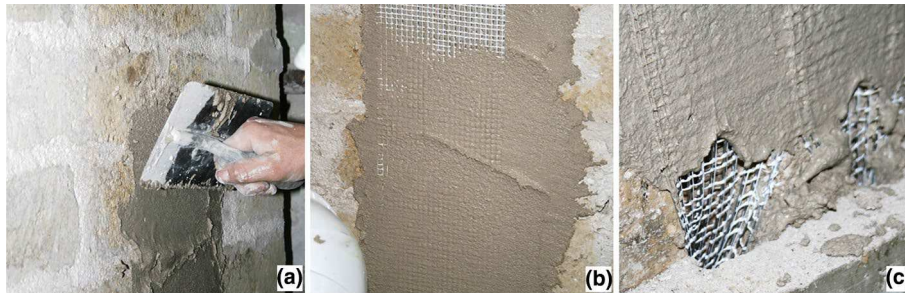
(a): laying of the first mortar layer (b): Installation of the steel textile (c): Steel connector and grout injection
