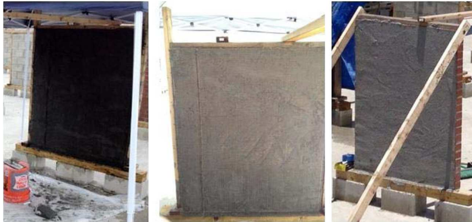
(a): first layer of mortar (b): precut carbon fabric (c): second layer of mortar
