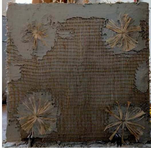
Fig. 7-14. HBW5 masonry wall upgraded with four jute diatons, 1x1 m 2 jute net (with mesh type 1.25cm x 2.5cm) and jute composite mortar (with 1% fiber (30mm) with respect to dry mortar mass).
