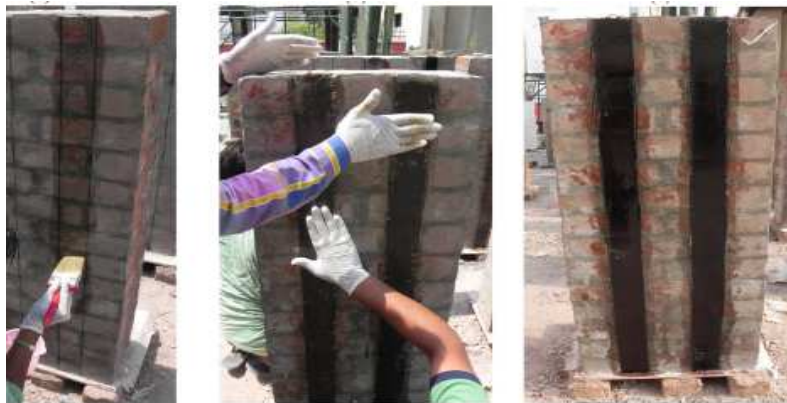
(a): Application of first layer of epoxy (b): Placement of BFRP strip (c): Application second layer of epoxy
