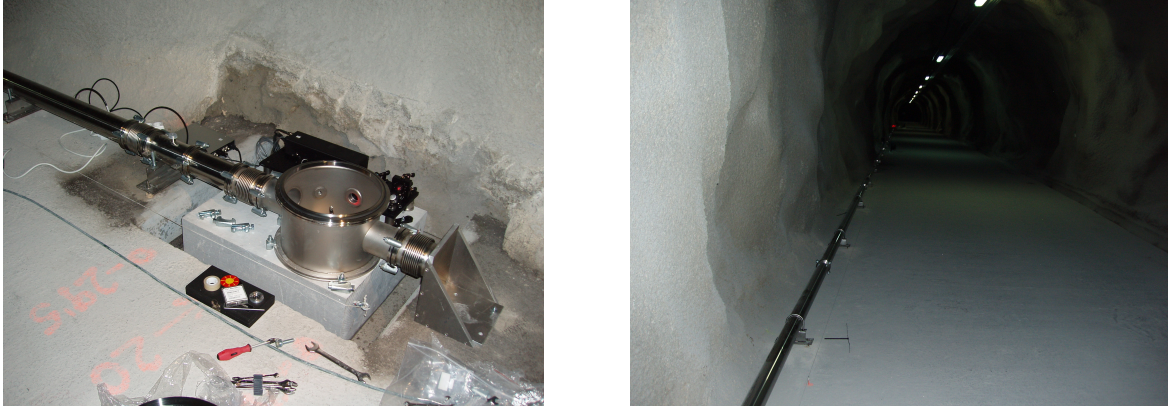
Figure 6.5: Main plinth (left picture) and vacuum line (right picture) in Bypass 16.
