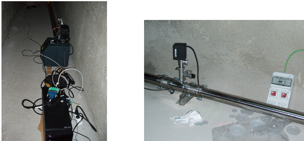
Figure 6.7: Vacuum pump (left picture) and electro-mechanical high vacuum valve (right picture) inside Bypass 16 and Laboratory 780, respectively.
