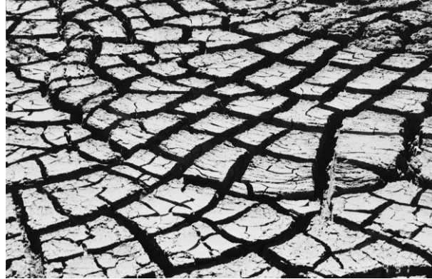
Figure 9.2 Cracking pattern in a desiccated soil surface (Blight 1997).
