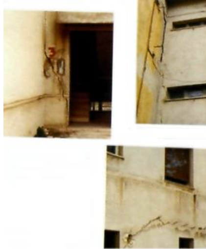
Figure 3.7 San Pietro in Guarano (Cosenza Province, Italy): damages to private houses (Antronico et al., 2003).
