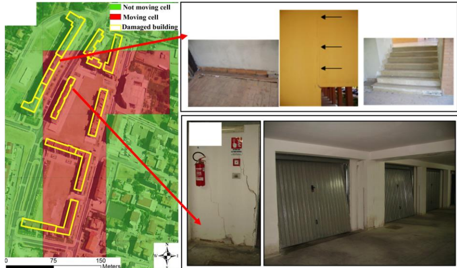
Figure 6.18 (a) Close view map of moving ENVISAT cells and damaged buildings in the municipality of Baronissi (Campania region, southern Italy); (b) damage recorded to infill walls and pavements; (c) damage recorded in the underground floor of a reinforced concrete building (Cascini et al., 2013a).
