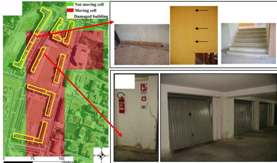
Figure 6.18 (a) Close view map of moving ENVISAT cells and damaged buildings in the municipality of Baronissi (Campania region, southern Italy); (b) damage recorded to infill walls and pavements; (c) damage recorded in the underground floor of a reinforced concrete building (Cascini et al., 2013a).
