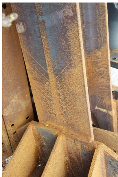
Figure 4.65 – Test 5: Yielding of the column bases
