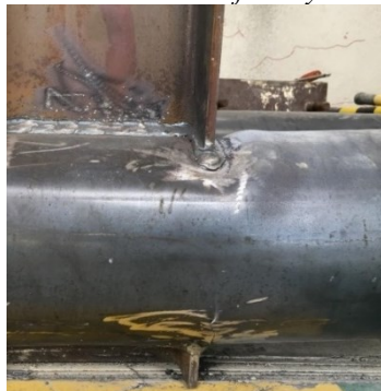
Failure mode of the specimen under cyclic loading
