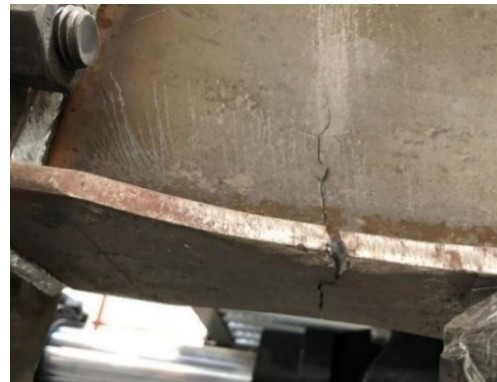
d) Failure at the centerline of RBS 1C
