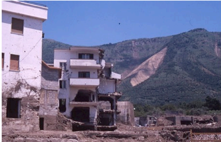
Figure 2-2. Example of damage caused by the impact of flow-like landslides in the Sarno area, Campania, southern Italy, 1998 (from Mavrouli et al., 2014)
