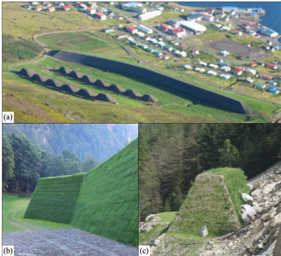
Figure 6-9. Some examples of MSE walls used as protection structures: a) Barbolini et al. (2009); b) Peila et al. (2007); c) Ronco et al. (2009).
